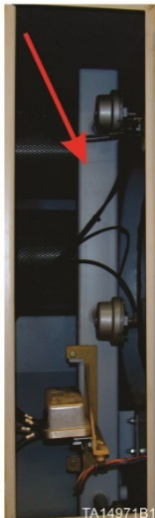
Figure 13. Compressed air manifold
