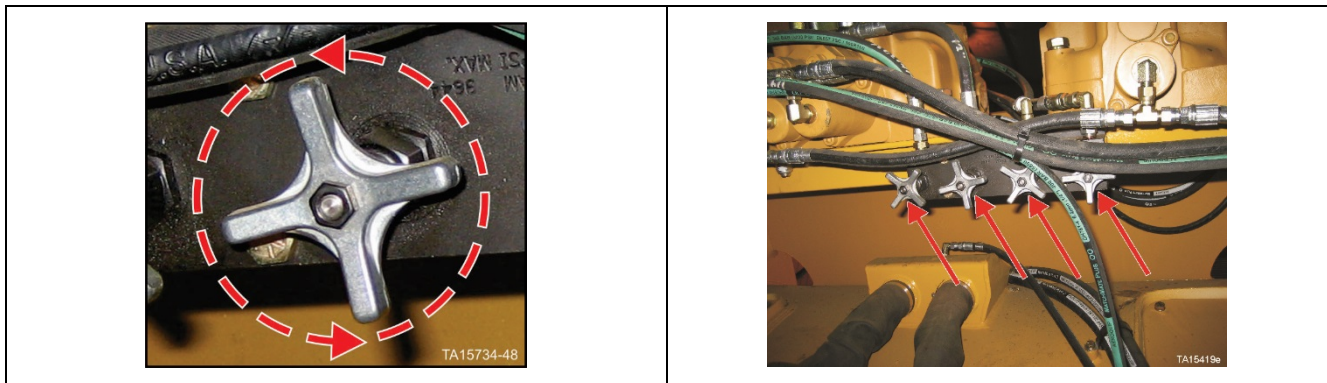
Figure 47. Pressure bleed down valves
