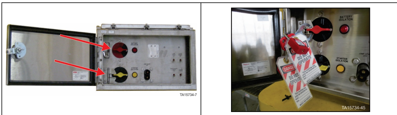
Figure 70. GEN 2 Isolation and Control Switches assembly – Battery isolation switch in OFF position with locks in place
