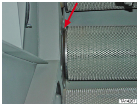
View through clean air chamber external door
