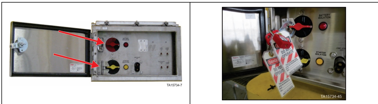
Figure 76. GEN 2 Battery Isolation Box – Battery isolation switch in OFF position with locks in place
